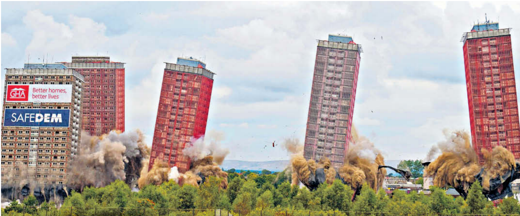
Road to demolition Glasgow's Red Road flats topple as they are demolished by controlled explosion. The tower blocks, which were a landmark on the city's skyline, were built in the Sixties to help solve a housing crisis, but quickly became associated with social breakdown, crime and vandalism. Thousands of people gathered yesterday to watch the destruction of the last remaining towers – although two stubbornly remained partially upright.
